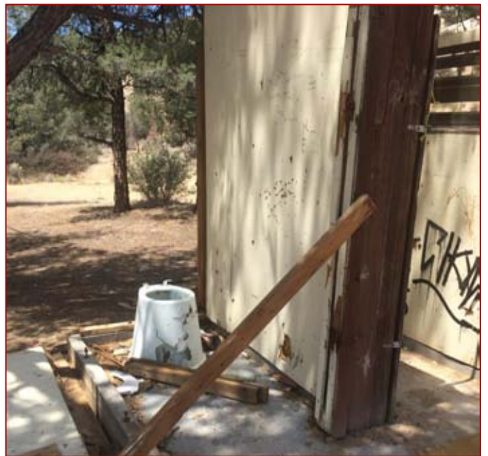
ABOVE, A BATHROOM IS VANDALIZED BY SHOOTING AND GRAFFITI AT A CAMPGROUND IN THE MOUNT PINOS RANGER DISTRICT. BELOW, A FORESTWATCH SURVEYOR RECORDS DATA AT A RESTROOM IN VENTURA COUNTY'S MOUNT PINOS RANGER DISTRICT, WHERE ENTIRE COLUMNS OF CONCRETE BLOCKS HAVE BEEN DESTROYED BY SHOOTERS.
